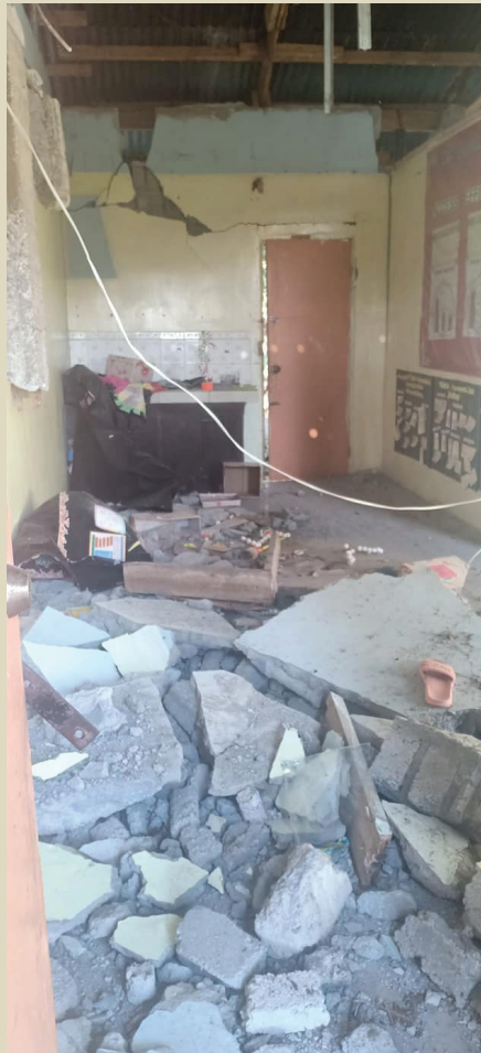
Homes and municipal structures were destroyed.
